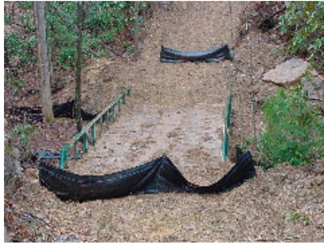
Bridge constructed to skid logs across a stream helps maintain high water quality.
